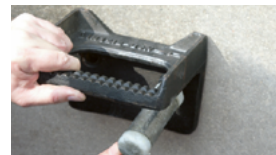
3. Place the step iron anchor through the hole in the step iron using the push-through method.
