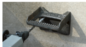
5. Drill and clean second hole. Step iron serves as plate drill jig.
